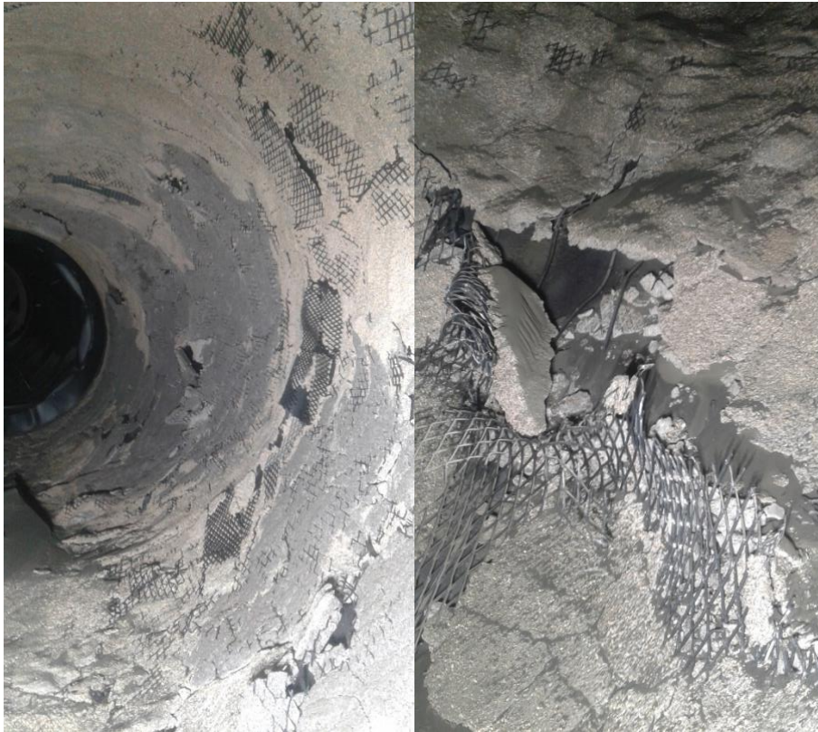
Figure 2: Inner sections of a damaged section of a WHR system due to wear and erosion in the Cement industry a) overall image and b) a more detailed image of damages [Courtesy of Cimsa Cimento].
