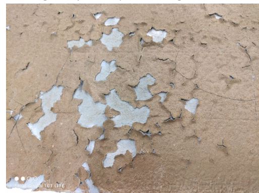
Damaged refractory, showing delamination.
